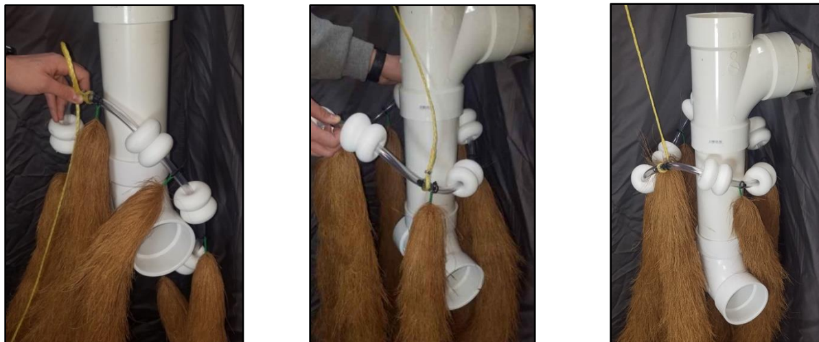
Figure 15, Bio-Brush Cluster Installed Around Outlet Housing
